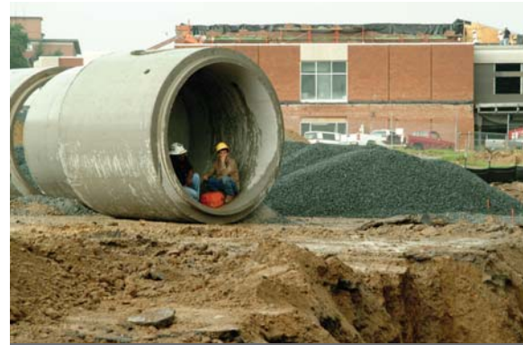
In the Antelope Valley, improvements such as channels, storm drains, and detention and retention basins are needed to control flood-prone areas in the region
