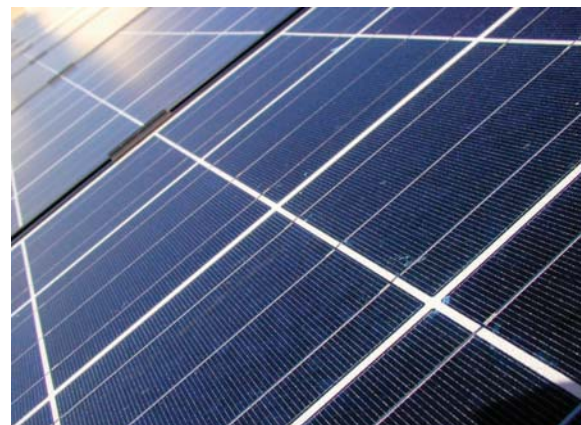
Through the use of energy saving devices like solar panels, proposed projects attempt to safeguard against both water and energy concerns in the Antelope Valley.
