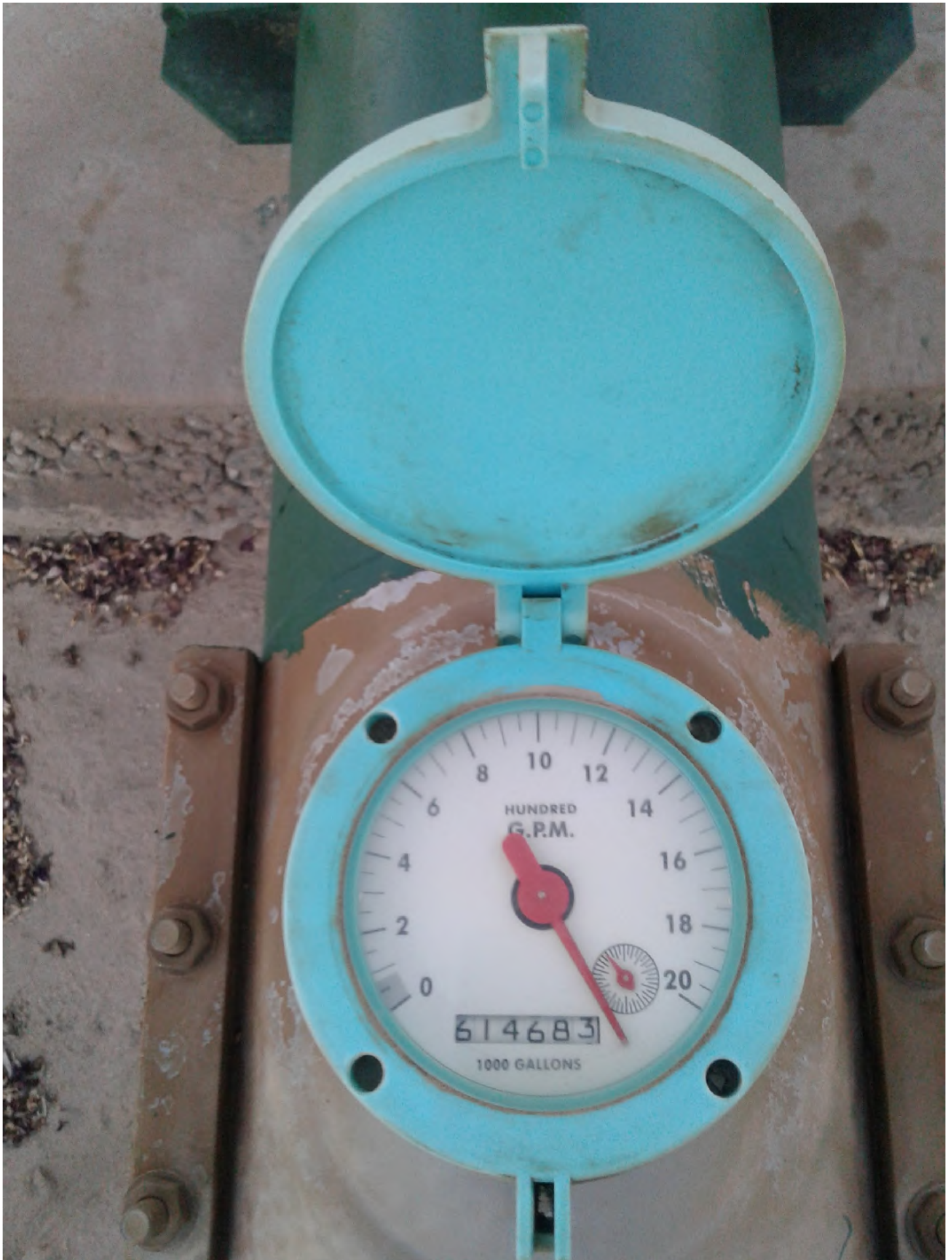
Treeland Antelope Valley Production Well # 3 (West), October 4, 2018
