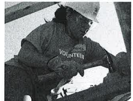
Theresa, an employee from the Planning division of Southern California Edison, volunteered to help build houses for Habitat for Humanity.
