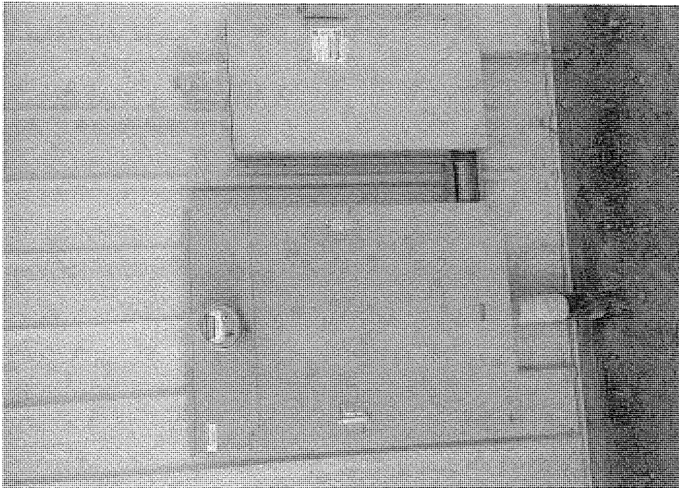
ZONE A EDISON CONTROL METER
